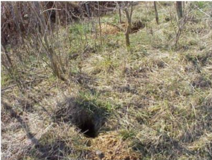
Figure M8.1: Animal burrow in pond embankment.
