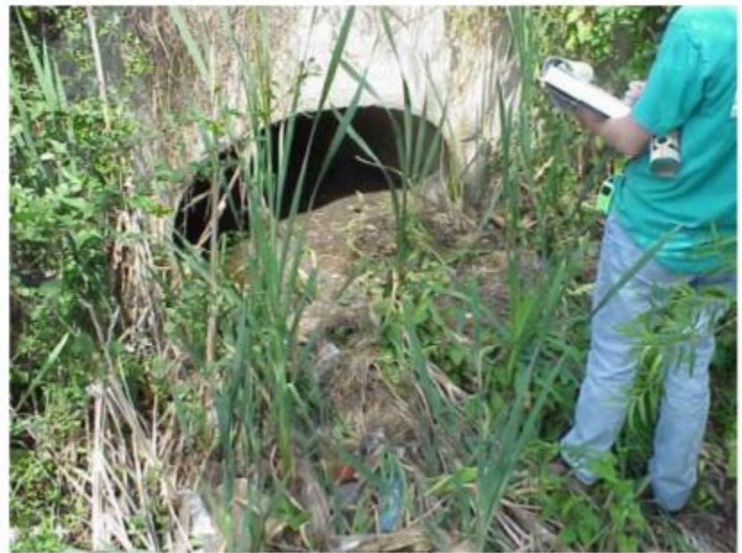
Figure M4.2: Excessive vegetation near an outfall.
